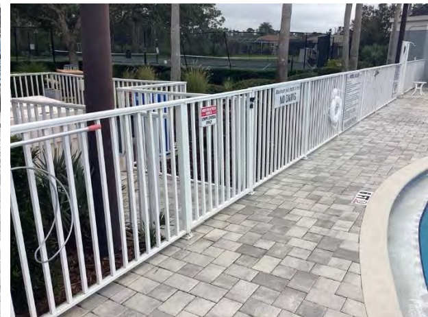
Aluminum fence overview
