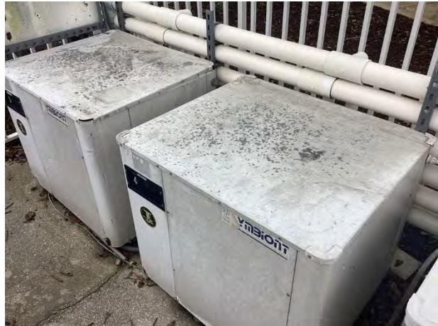
Geothermal heaters for near term
