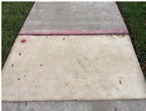
Sidewalk trip hazard
