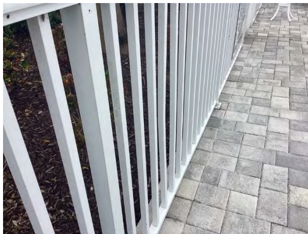
Fence picket damage
