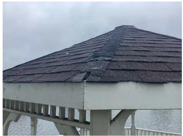
Shingle roof damage
