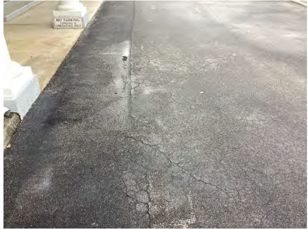
Pavement cracks - Clubhouse
