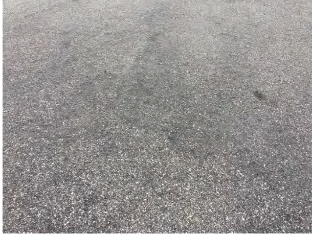
Pavement raveling - Savannah Drive
