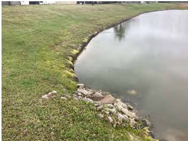
Pond N shoreline previous repairs
