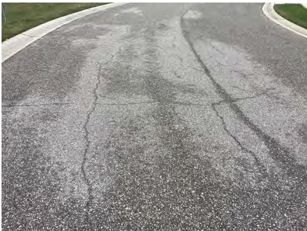
Pavement cracks - Jonah Drive
