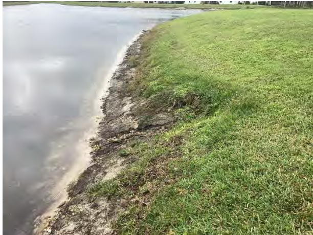
Extensive shoreline erosion Pond P
