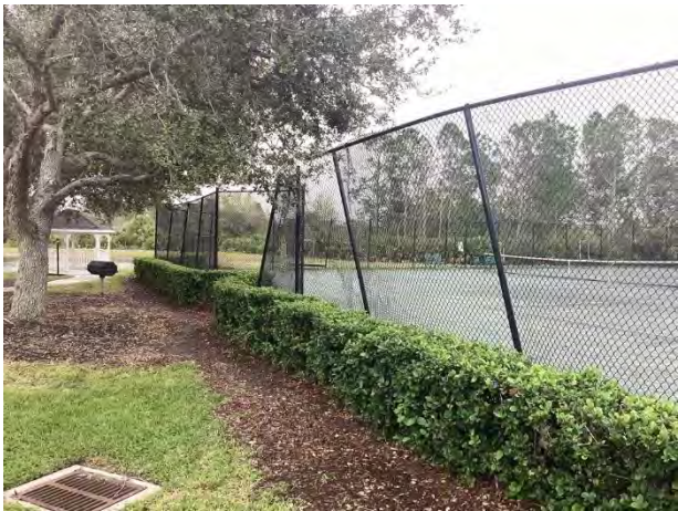
Fence leaning section
