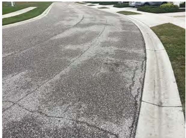
Pavement cracks - Jonah Drive
