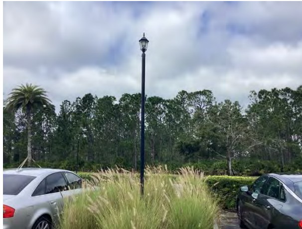
Light pole and fixture
