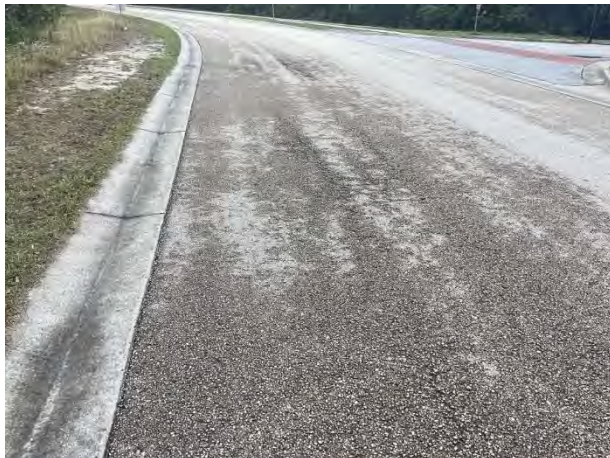
Pavement cracks – Sycamore Drive
