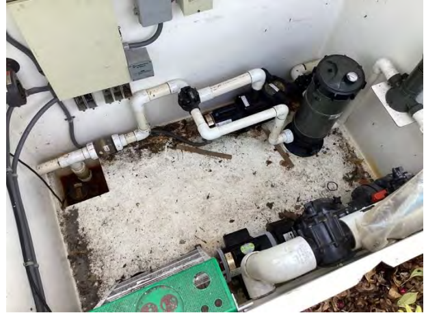
Mechanical equipment overview
