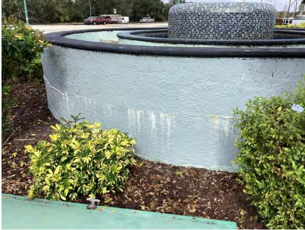
Stucco cracks and stains
