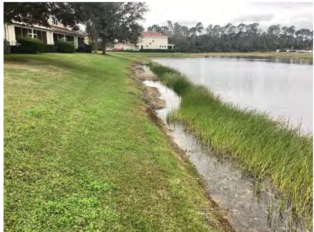
Minor shoreline erosion at Pond B
