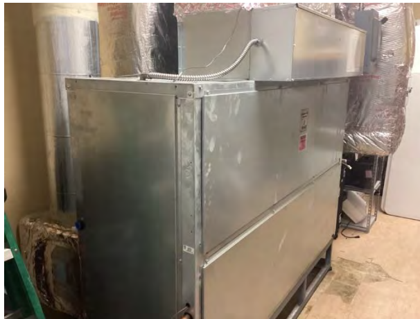
New air handling unit
