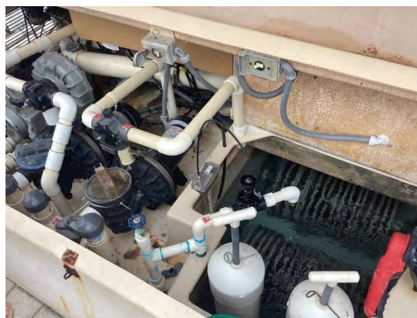
Pool mechanical equipment overview
