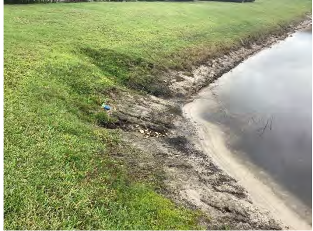
Extensive shoreline erosion Pond P
