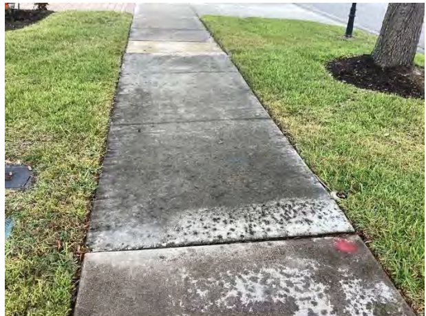
Sidewalk trip hazard
