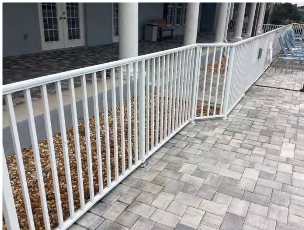
Aluminum fence overview
