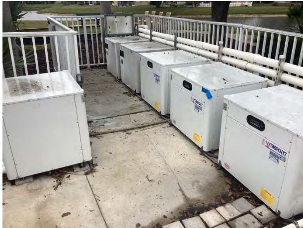
Geothermal heater overview
