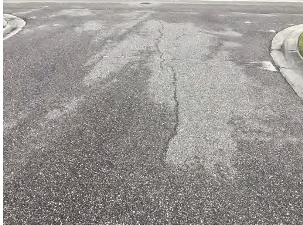
Pavement cracks - Boxwood Street
