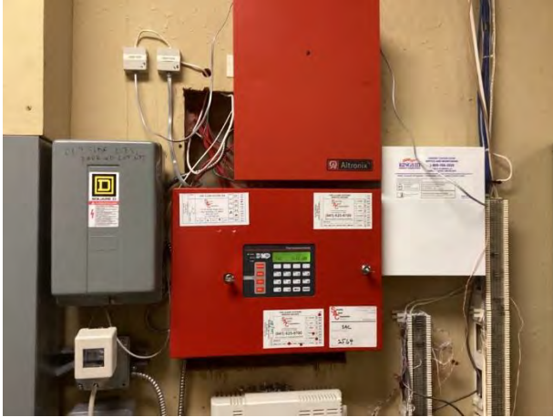
Control panel overview
