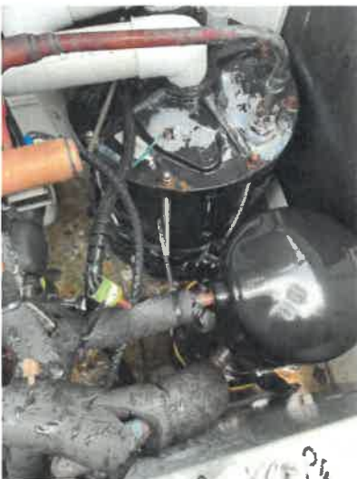
Picture D. Pool Heaters
