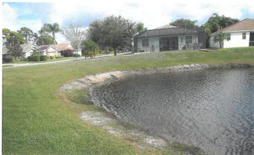
Figure 12: Lake 14 - Exposed MES and erosion along north bank.
