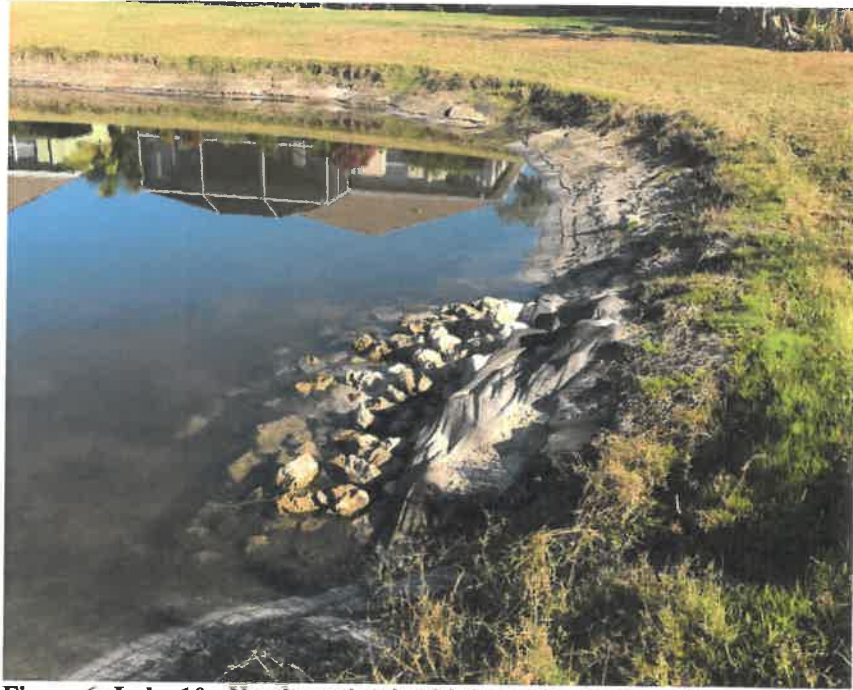
Figure 6: Lake 10 - Northeast bank with 2 erosion sites needing repair.
