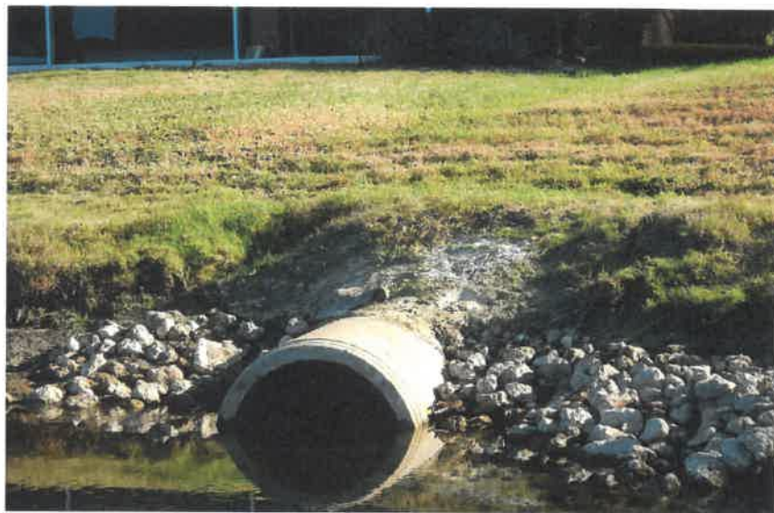
Figure 8: Lake 11 - Exposed pipe.
