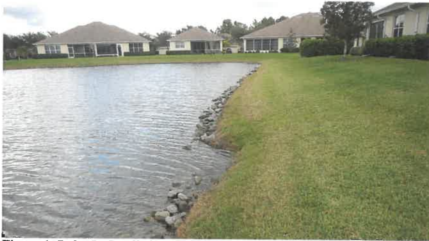
Figure 1: Lake 5 - Small rip-rap repair required along the east bank.
