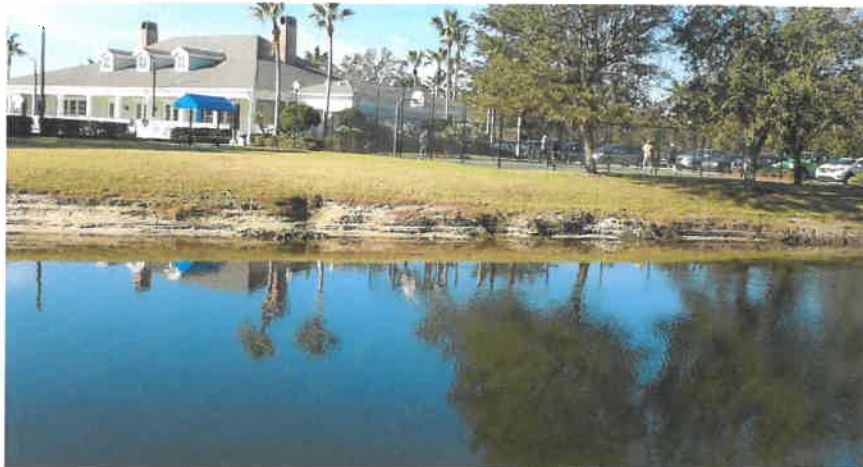
Figure 5: Lake 10 – Erosion along the southwest bank at the clubhouse.
