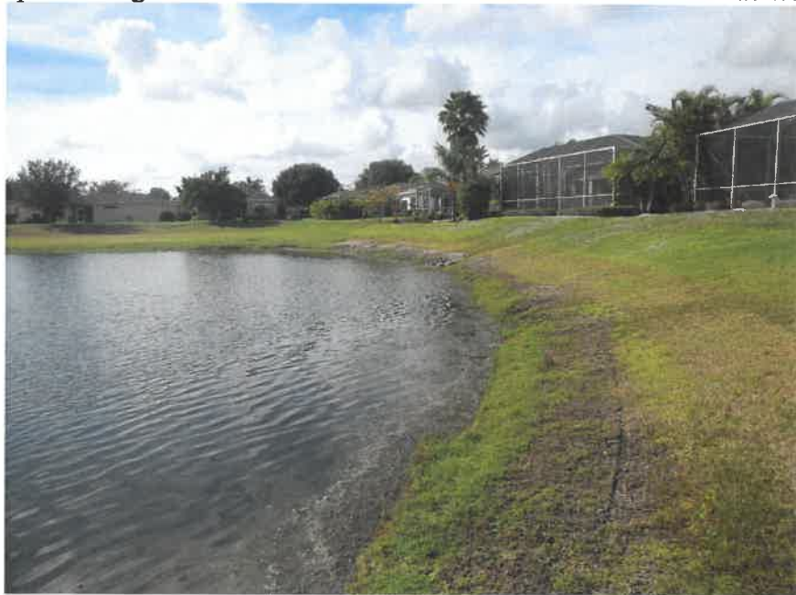
Figure 10: Lake 13 – Erosion along the north bank.
