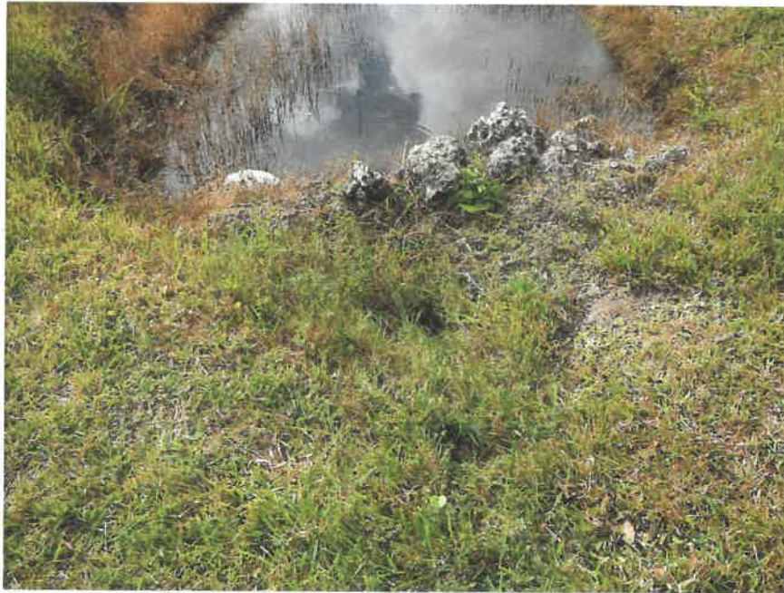
Figure 3: Lake 8 – Erosion at the north culvert.
