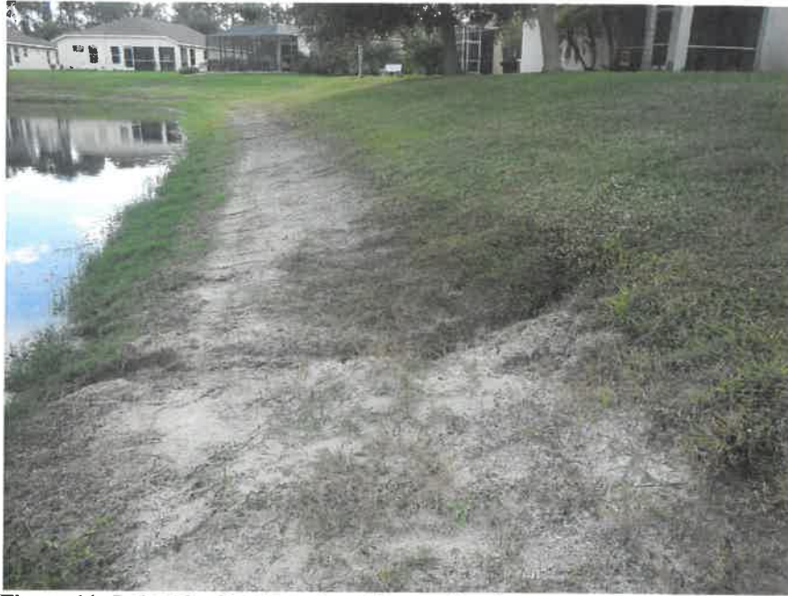
Figure 11: Lake 13 – Erosion along the west bank.
