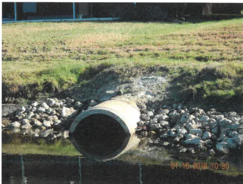
Figure 6: Lake 11, Photo 27, Add new rip-rap on top of exposed pipe
