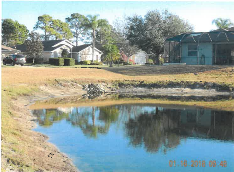
Figure 7: Lake 14, Photo 19, Exposed piping needing more rip-rap
