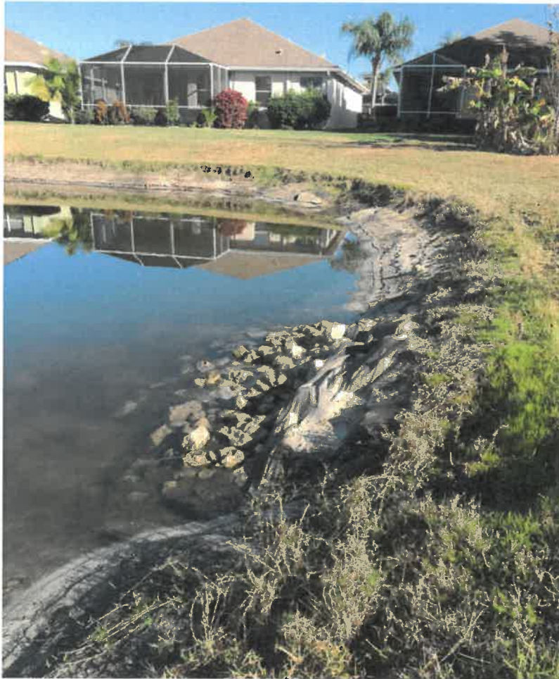
Figure 4: Lake 10, Photo 8 Northeast bank with 2 erosion sites needing repair
