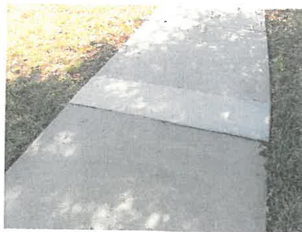
Concrete sidewalk with previous repair
