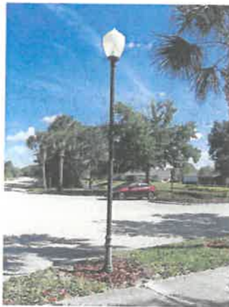
Light pole and fixture
