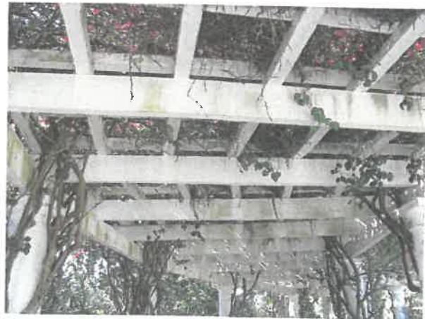
Biological stains at wood arbor
