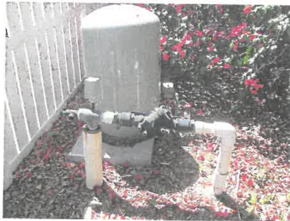
Irrigation well and pressure tank
