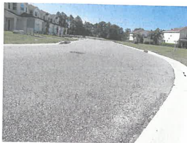
Asphalt pavement edge deterioration at the Towns
