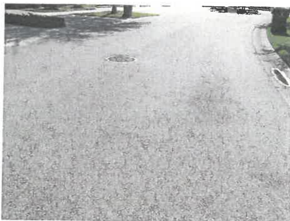
Asphalt pavement with early stages of raveling
