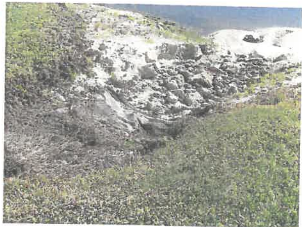
Pond D - erosion at canal inlet
