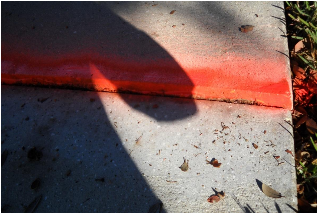
Pictures of Sidewalk repairs needed
