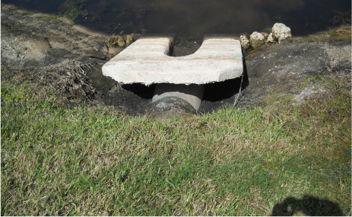
One of the mitered ends in need of attention.
