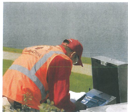
Entering smart controller parameters
