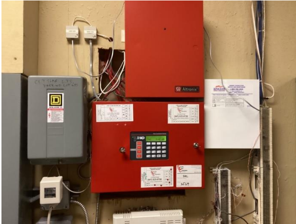
Control panel overview
