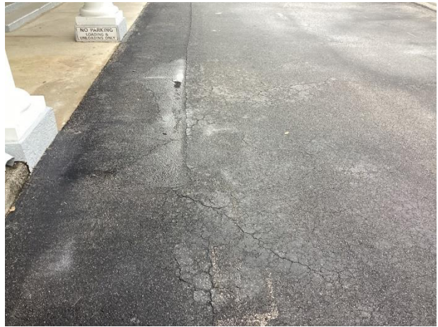
Pavement cracks - Clubhouse
