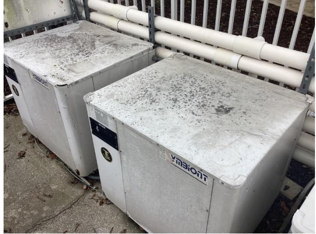
Geothermal heaters for near term
