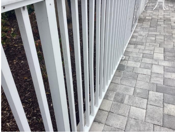
Fence picket damage
