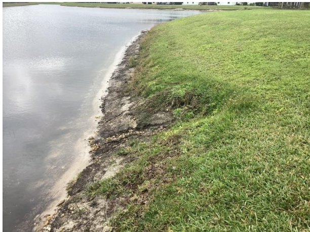
Extensive shoreline erosion Pond P
