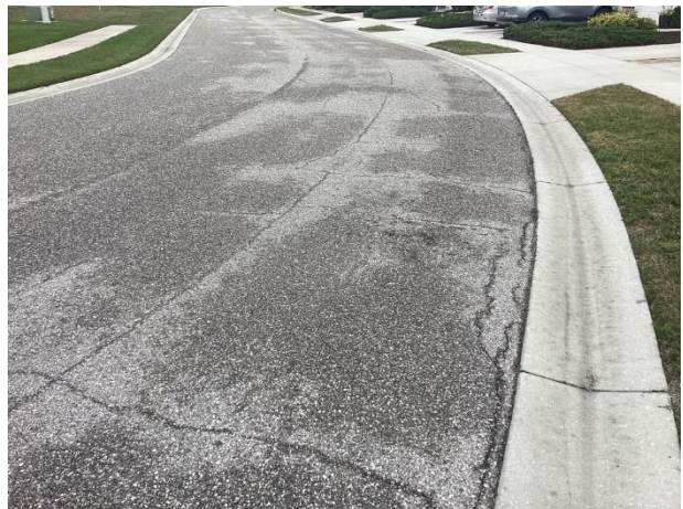
Pavement cracks - Jonah Drive
