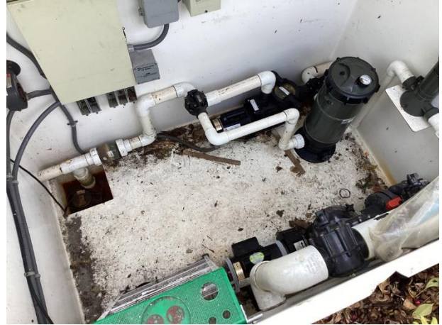
Mechanical equipment overview
