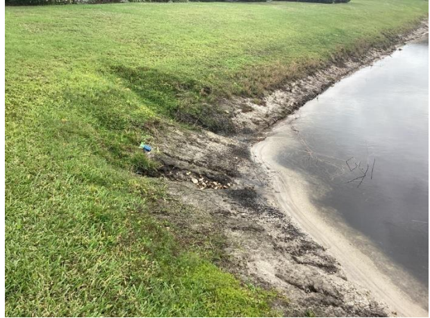
Extensive shoreline erosion P
