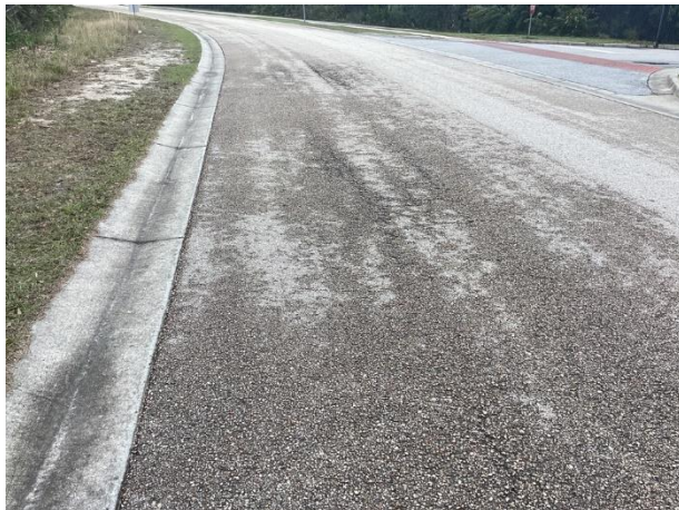
Pavement cracks – Sycamore Drive
