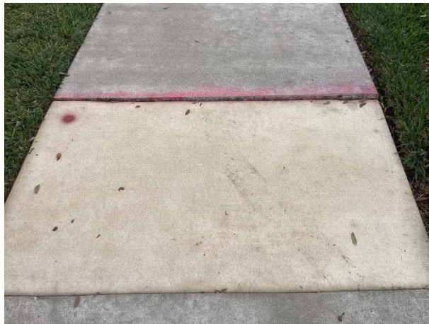
Sidewalk trip hazard
