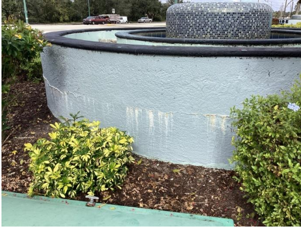
Stucco cracks and stains
