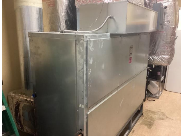
New air handling unit
