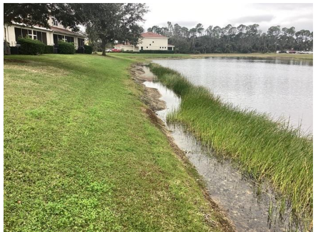
Minor shoreline erosion at Pond B
