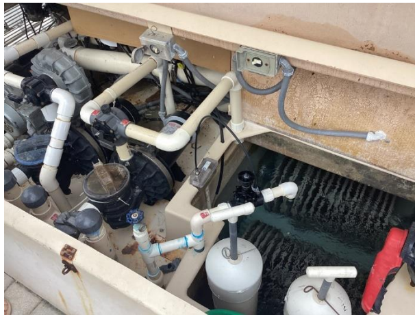
Pool mechanical equipment overview
