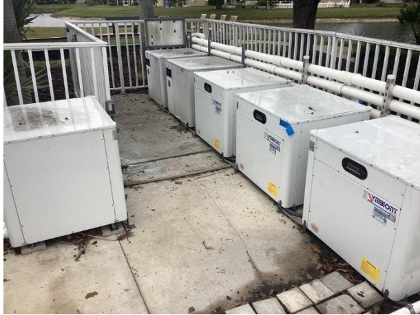
Geothermal heater overview
