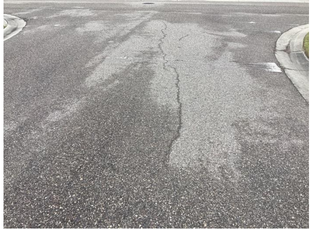
Pavement cracks - Boxwood Street
