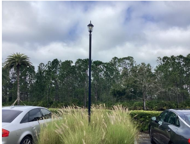
Light pole and fixture
