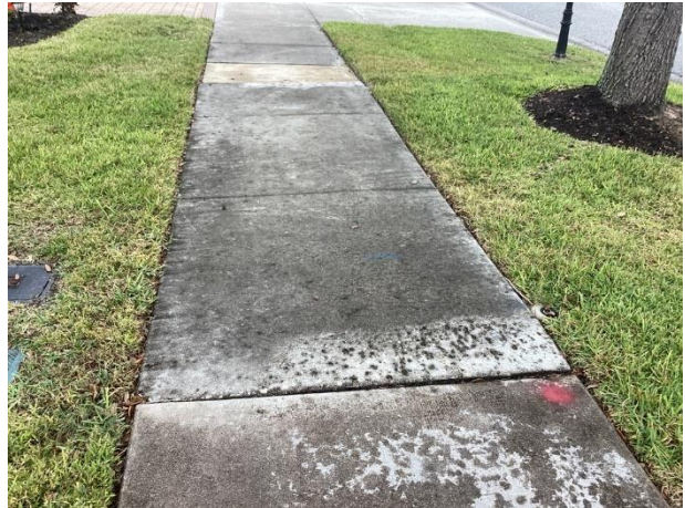
Sidewalk trip hazard
