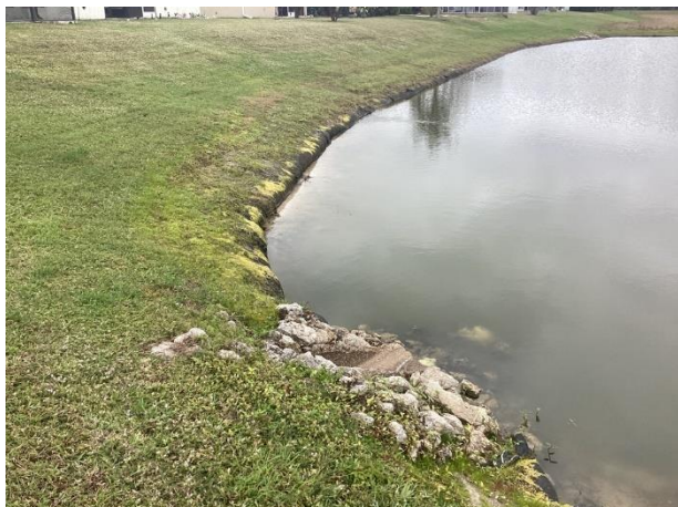
Pond N shoreline previous repairs
