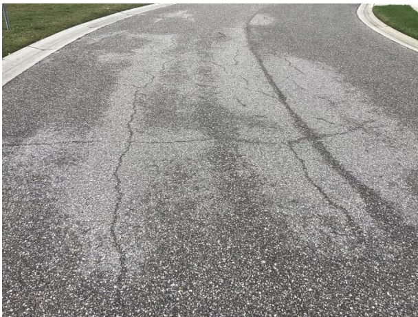
Pavement cracks - Jonah Drive
