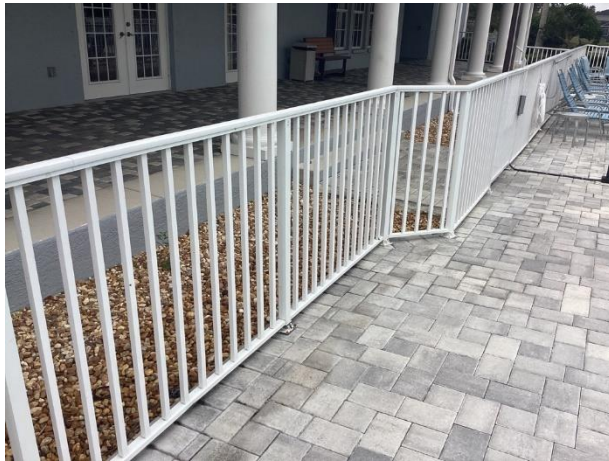
Aluminum fence overview
