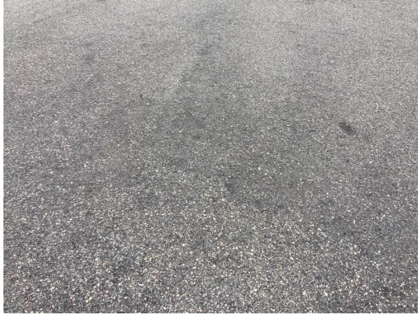
Pavement raveling - Savannah Drive
