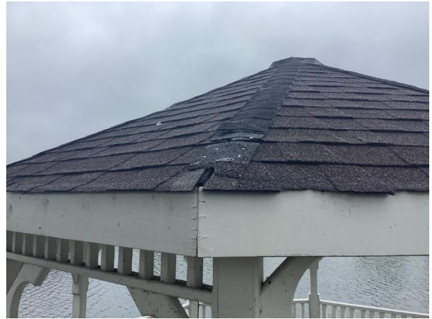
Shingle roof damage
